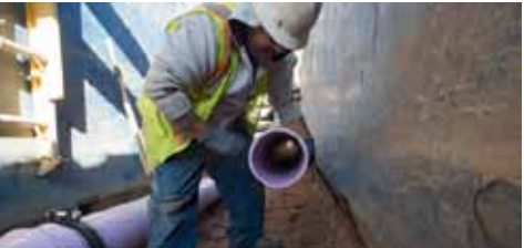
Recycled water from a "purple pipe" system will heat and cool the facility with geothermal energy.
